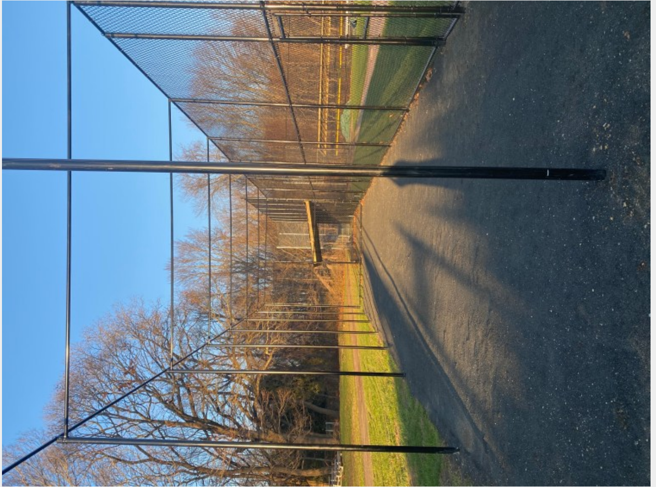
Initial building is taking place for the new 50/70 baseball field in Easton (Photo: Rob McDermott)
