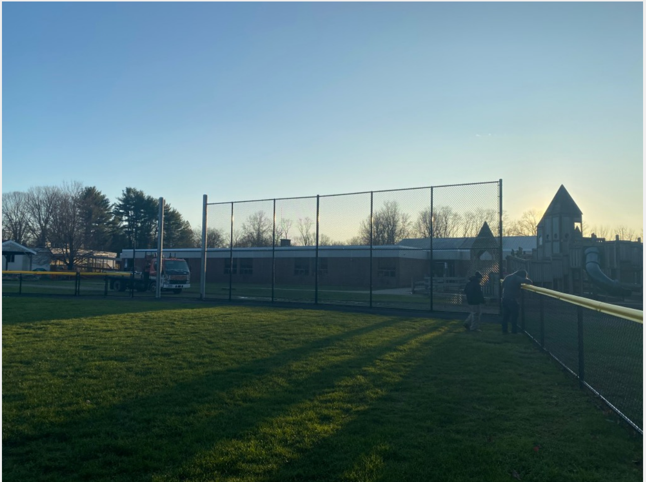
Initial building is taking place for the new 50/70 baseball field in Easton (Photo: Rob McDermott)
