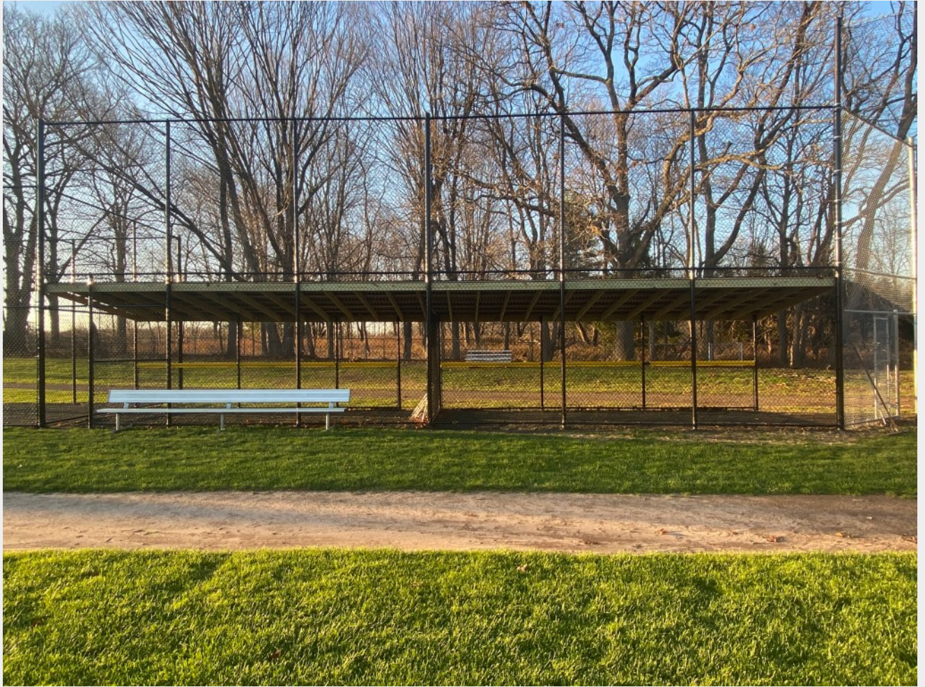
Initial building is taking place for the new 50/70 baseball field in Easton (Photo: Rob McDermott)
