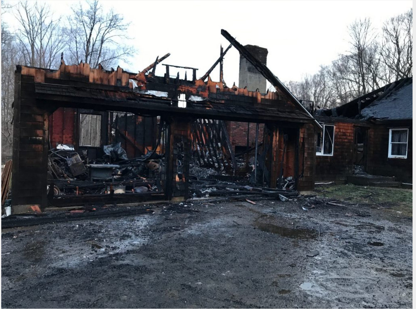
• The house at 330 Rock House Road was a total loss and is inhabitable. — Photo Courtesy of Easton Police Department
